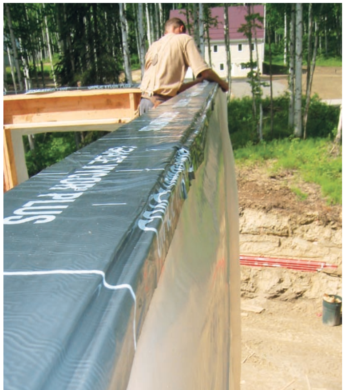
Figure 2. The author's crew applies a 9-inch-wide peel-and-stick flashing to the top plates, adhering it to the inside edge of the plates (top) and lapping it onto the 6-mil poly membrane on the sheathing (above).
