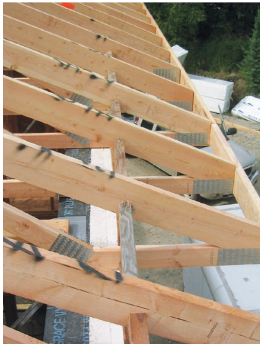
Figure 5. To ensure the continuity of the barrier membrane and exterior insulation, the wall to the right of this garage roof was covered with poly and foam before the roof was framed (top). Moving truss blocks in line with the outer edge of the exterior EPS will allow the cellulose in the attic to completely cover the full thickness of the exterior walls (above).
