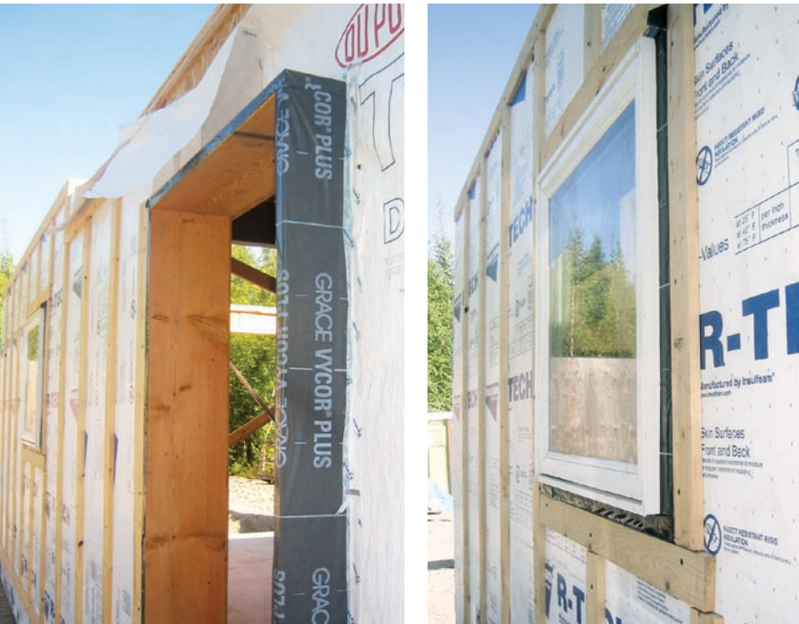
Figure 4. On past jobs, the author installed windows at the face of the wall by setting them in solid lumber bucks protected with peel-and-stick flashing (top). The bucks are attached to the inside of the rough opening and taped or flashed to the wall membrane (above left). Bucks are sized so that when foam insulation and furring are installed, the siding will be in the proper plane (above right).
