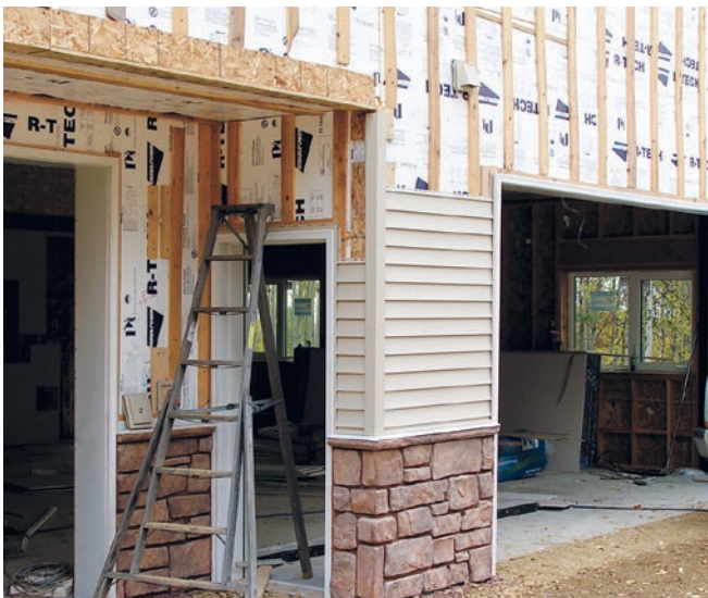
Figure 6. The EPS insulation is first tacked in place, then secured with long screws fastened through furring strips into the framing (top left). Wide furring members are needed at corners (top right) and around openings (above) to provide backing for trim.
