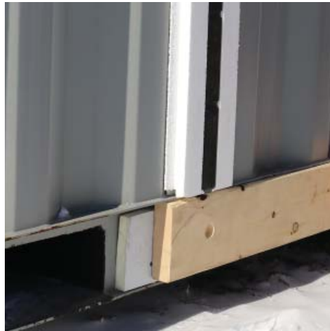
Option two for insulating and furring out the beam.
